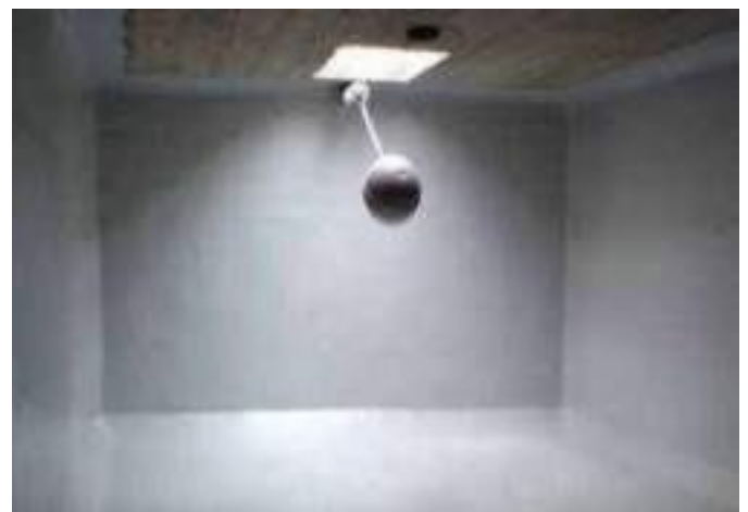
SEWAGE TANK – IBRI
